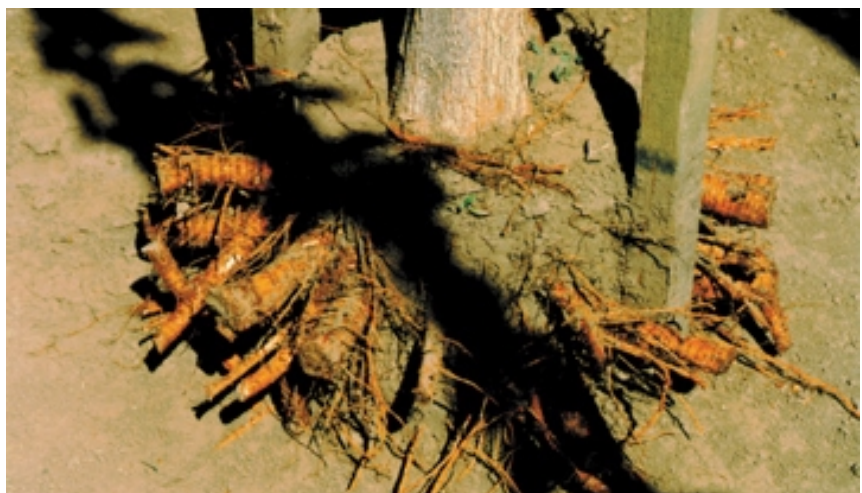
The photo above of a control tree without barrier illustrates the surface buttress roots that cause damage to hardscapes.
